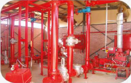
Agiba Sites Fire Pumps
