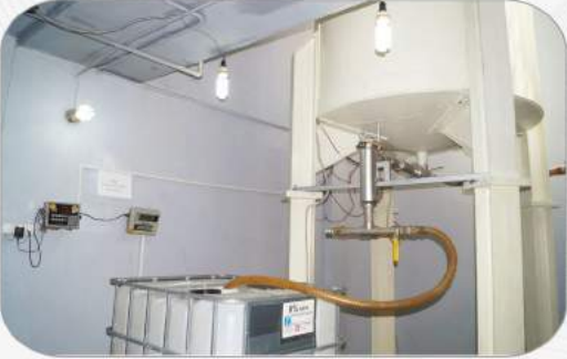
UL Listed foam blending station
