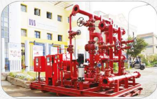
UL/FM pump skid project
