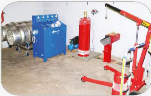
LPCB - FM200 filling station & systems
