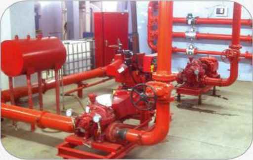
UL/FM fire pumps test rig
