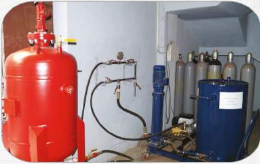
Hydrostatic pressure test station
