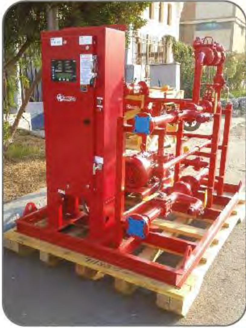
Foam Pump Skids
