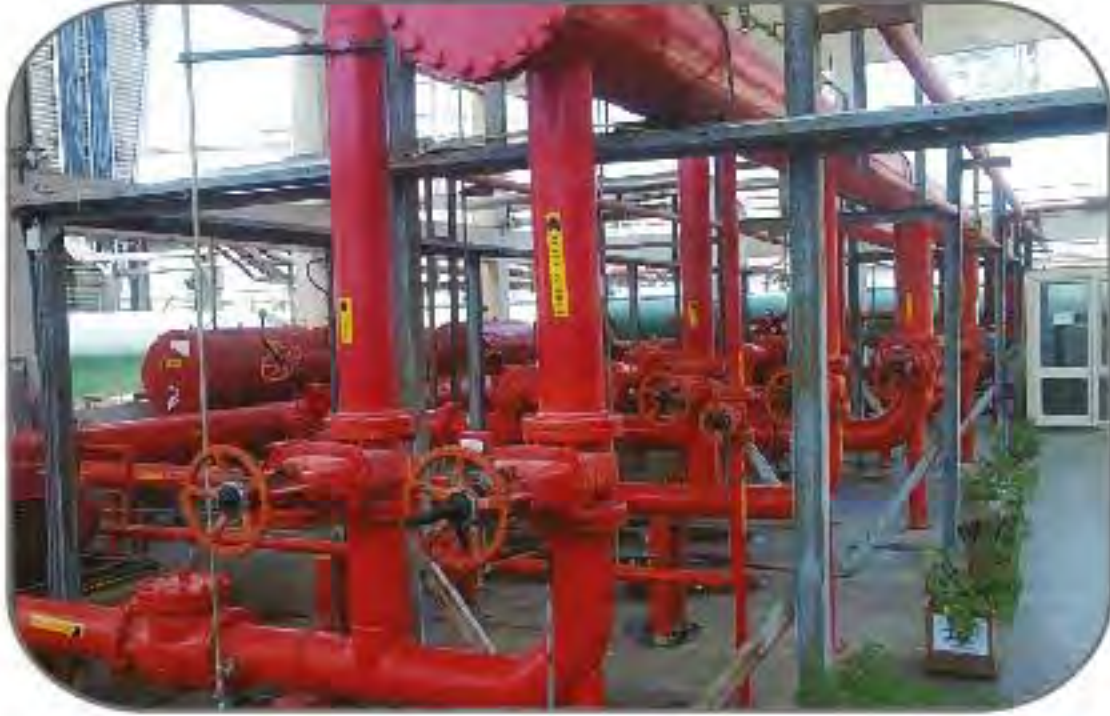
18000 gpm- Fire Fighting Pump Station consists of 3x 5000 gpm Diesel Pumps and 2x1500 gpm Electric pumps.
