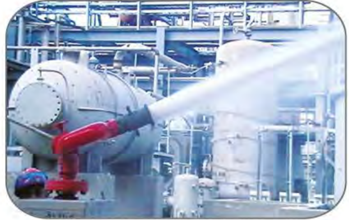
Water & Foam Monitors around the whole Factory.
