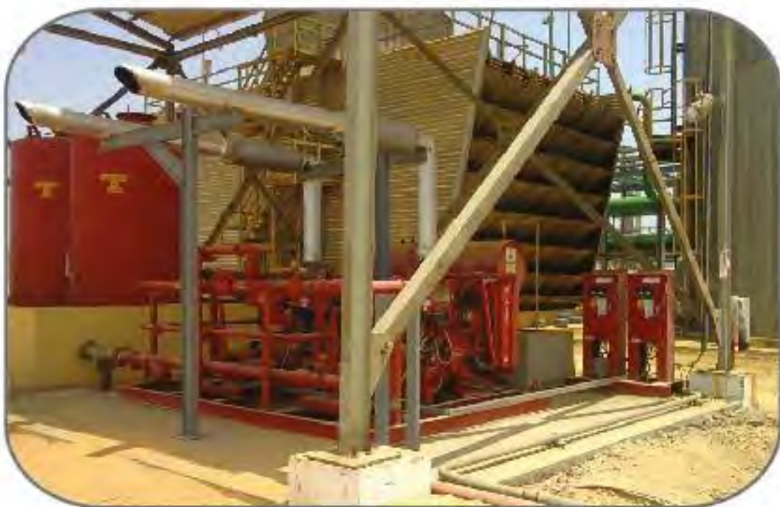
2x Foam Pump Stations ,one with 2 x electric foam pumps skid unit and 2 x diesel foam pumps skid unit , each with 20 m3 - 3%AR-AFFF foam concentrate in two atmospheric tanks.
