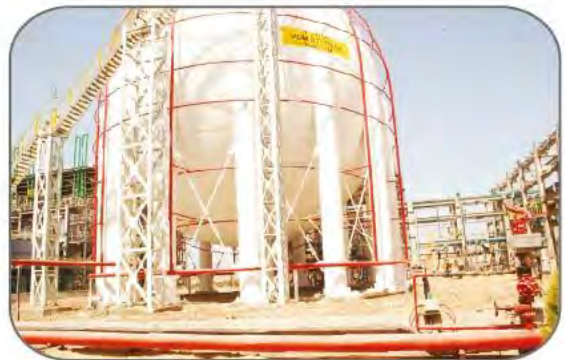
Manual and automatic operation of a cooling System for VCM-Pressurized gas spheres..
