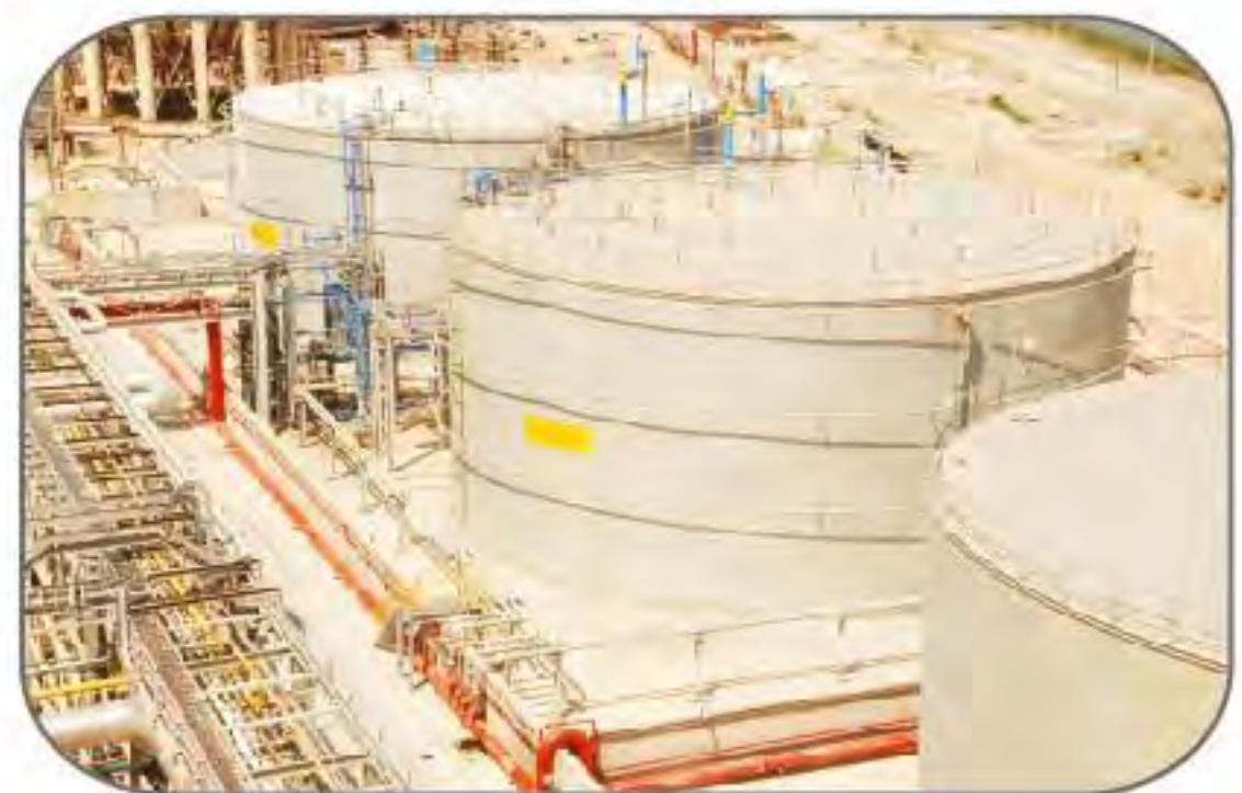
Manual and automatic operation of a Fire Protection system using (water/foam) systems for EDC and Methanol Tanks.
