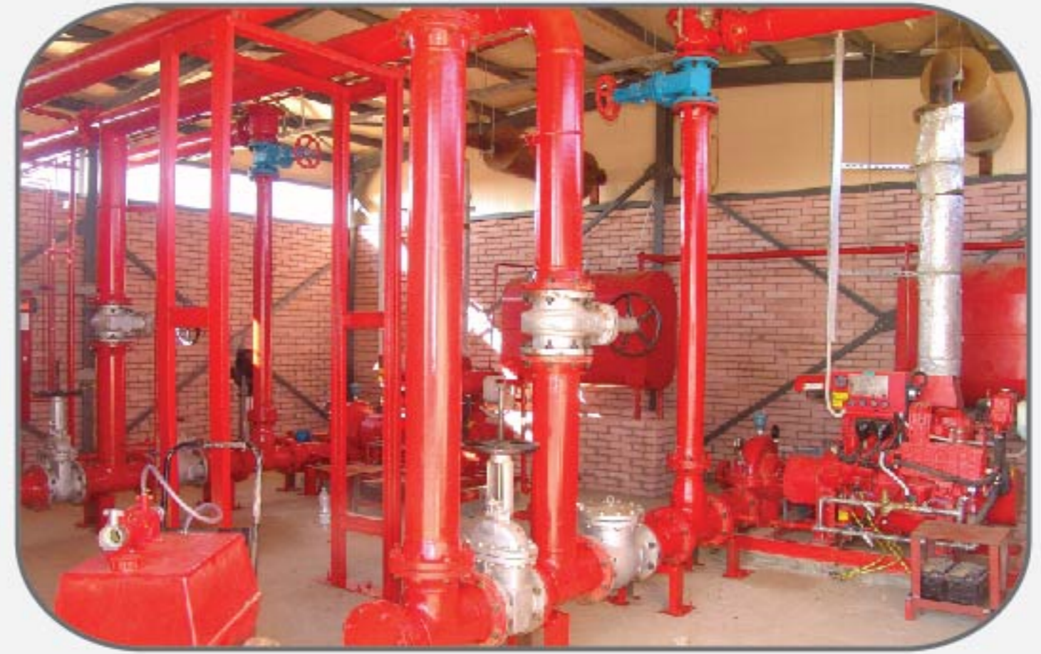
AGIBA SITES FIRE PUMPS
