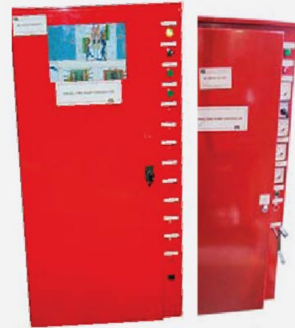
Floor stand Fire Pumps controllers as per NFPA20.
