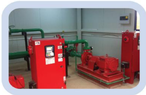
Romania - Power Station
