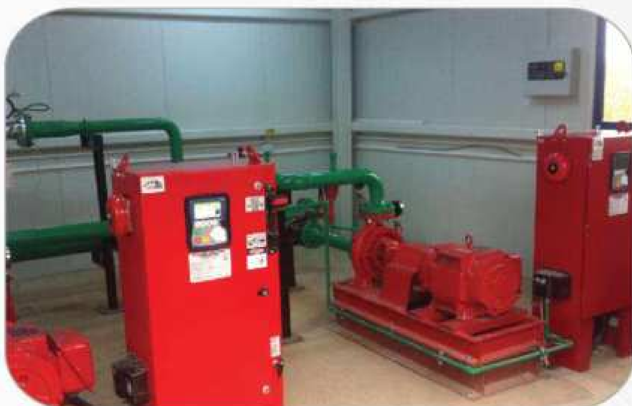
Romania - Power Station
