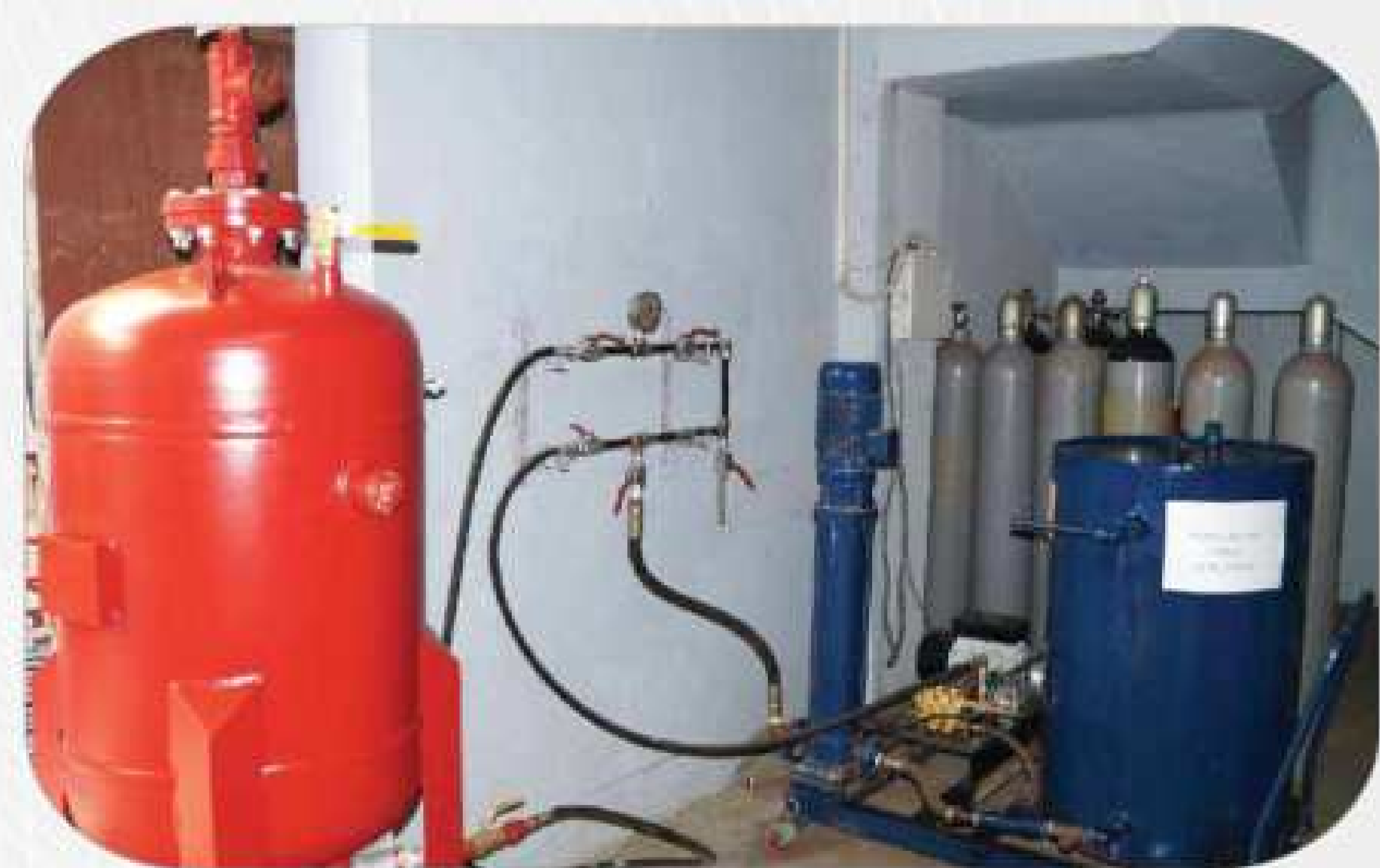
Hydrostatic pressure test station
