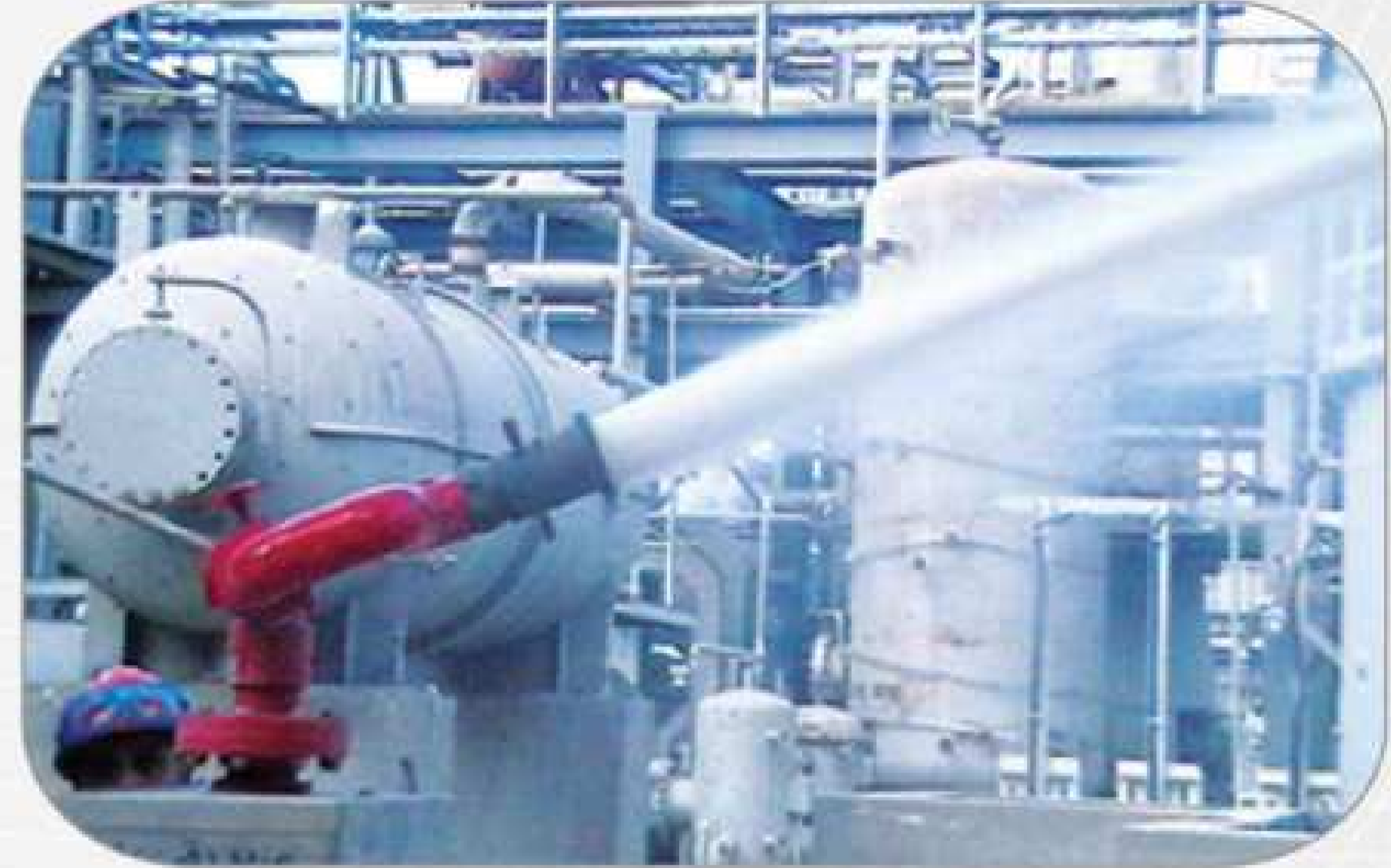
Water & Foam Monitors around the whole Factory.
