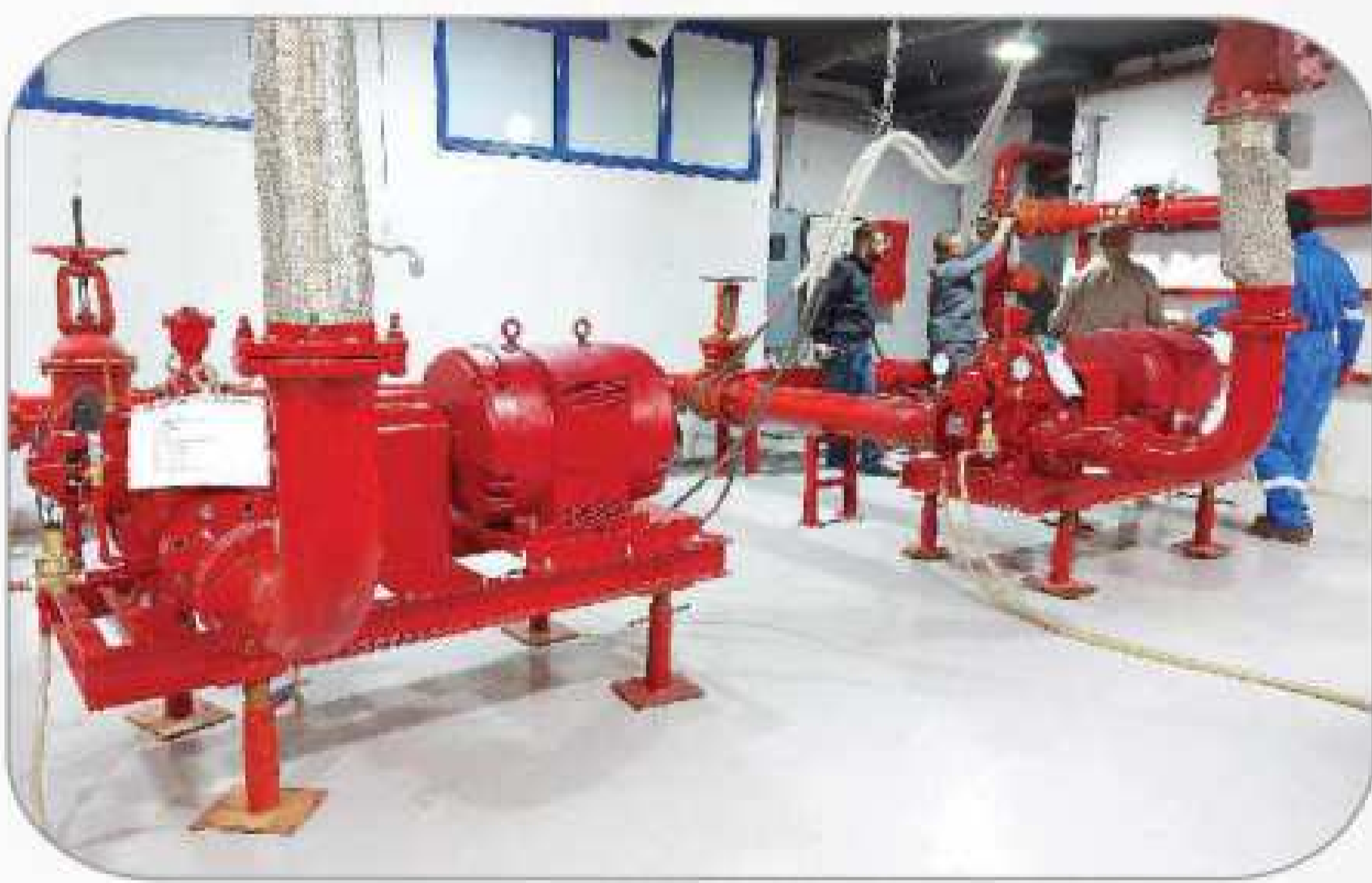
UL/FM fire pumps test rig
