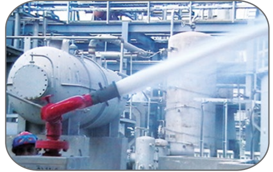
Water & Foam Monitors around the whole Factory.
