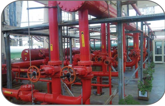
18000 gpm - Fire Fighting Pump Station consists of 3x 5000gpm Diesel Pumps and 2x 1500gpm Electric pumps.
