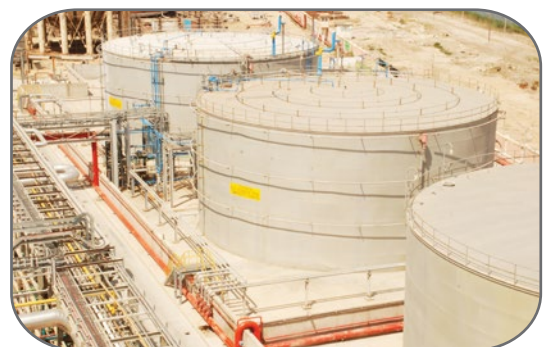
Manual and automatic operation of a Fire Protection system using (water/foam) systems for EDC and Methanol Tanks.
