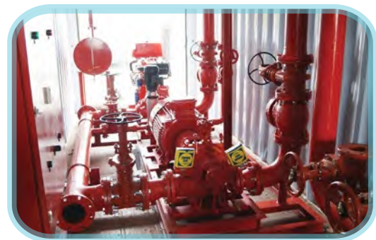
EL - SEWEDY ELECTRIC (ELECTRIC POWER STATION)
