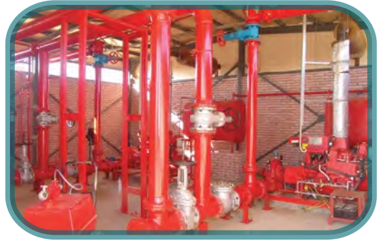
AGIBA SITES FIRE PUMPS
